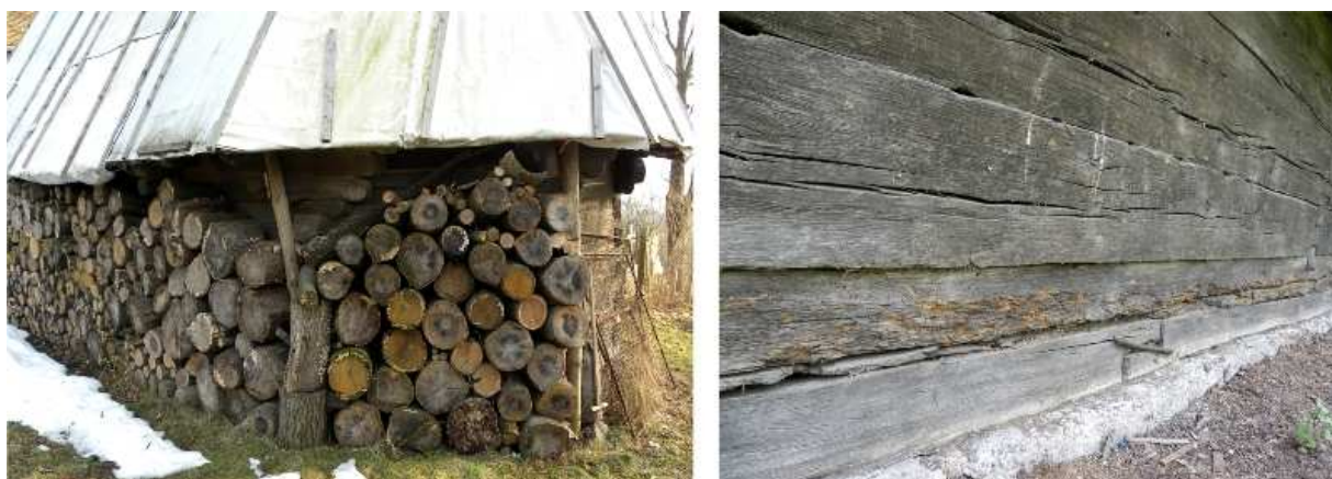
Fig. 5 – a. Wooden pieces stored on the walls; b. Biological attack at the beams
